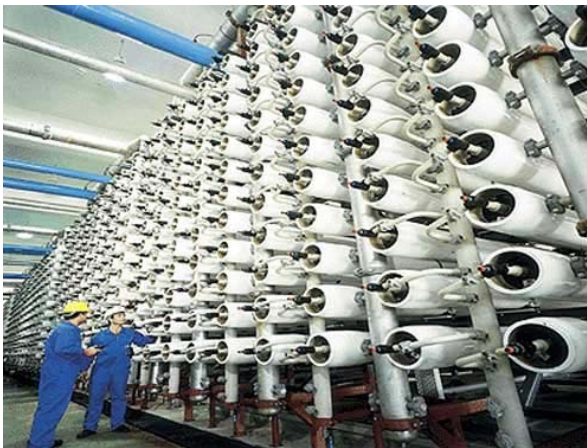
A bank of some of the 38,000 cylinders containing spirally coiled membranes in the largest sea water reverse osmosis plant in the world at Ashkelon on Israel's Mediterranean coast. The plant produces 100M m^3 /year, 5+% of Israel's total water need.
